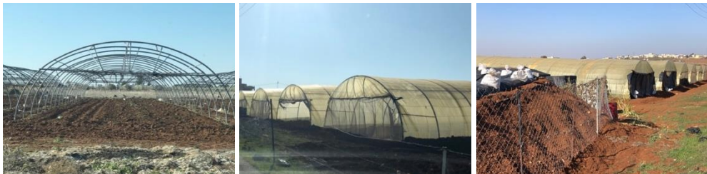
Figures 3, 4 & 5: Construction of 'green houses' at planting time - during the growing season with rainwater storage
